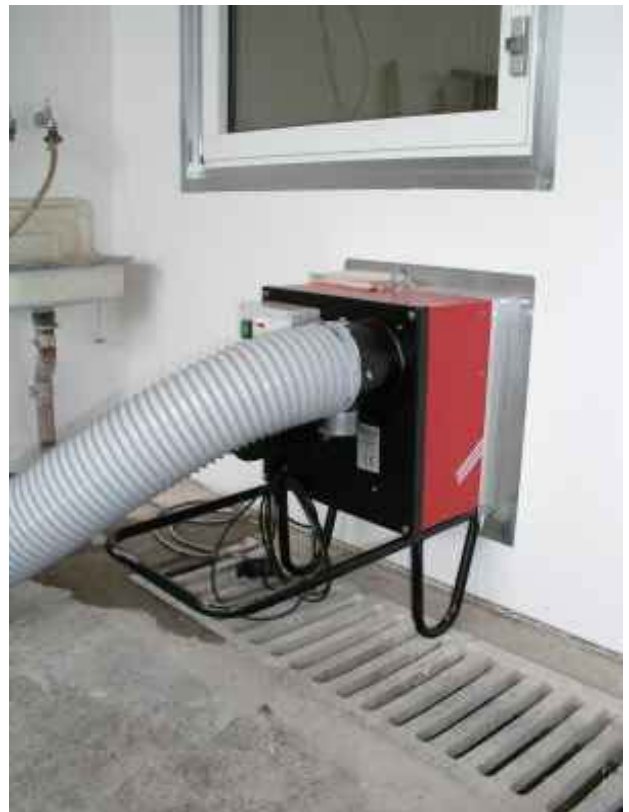
fig. 5.3 - 8 One of the two high-performance ventilators
